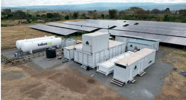
Anhydrous ammonia fertilizer plant at Kenya Nut Company. Photo: Talus Renewables.
